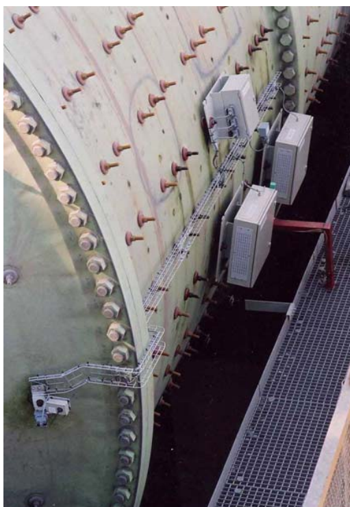
Figure 12: Example of Sensomag® installation on the mill shell
