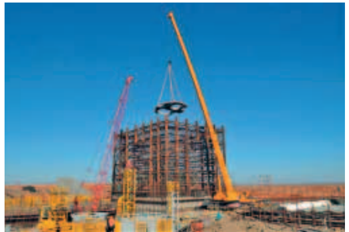
Preparation for sinking platform installation at Oyu Tolgoi #2 (Top) and installation of the platform (Bottom)
