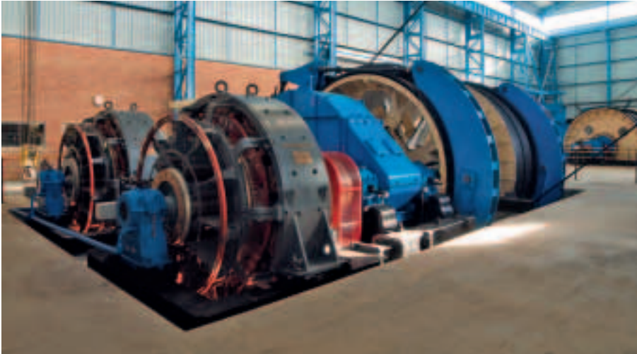
DRATS two refurbished hoists at Great Basin Gold's Burnstone gold mine
